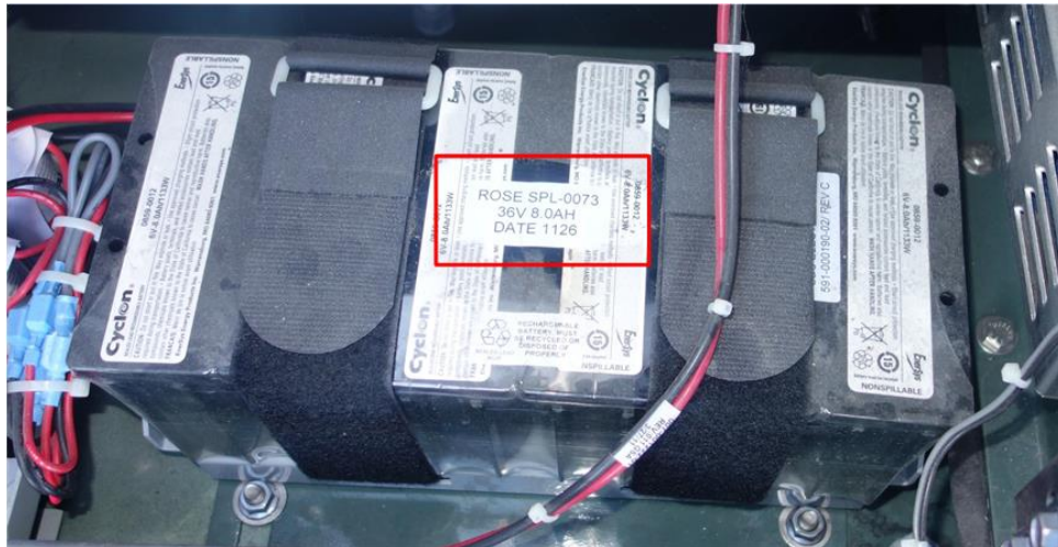
Figure C.1a. Remote Supervisory Battery Pack
