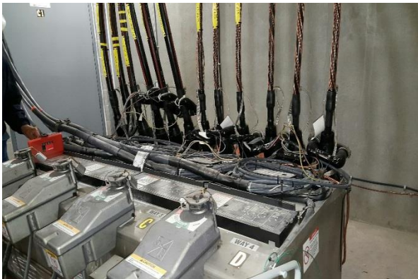
Figure 4.2.2a. Switch in In-Building Vault
