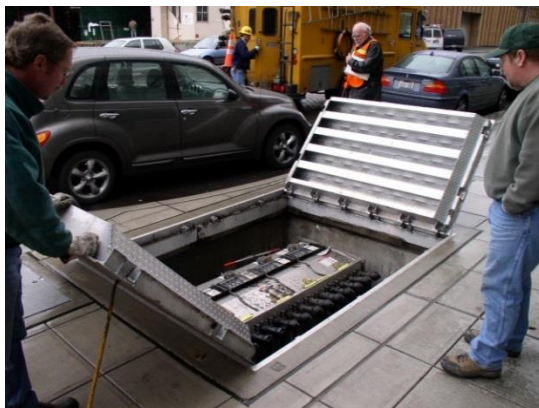
Figure 4.1.3. Switch in Wet, Subsurface Vault
