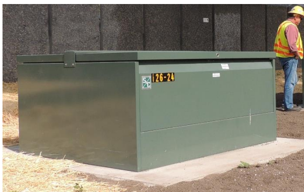
Figure 4.1.1. Manually Controlled Padmount-Style Switch
