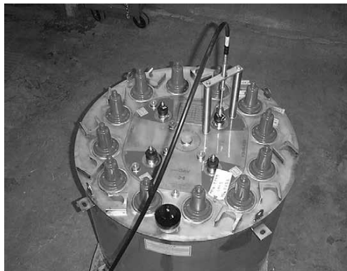
Figure 6. VACop IV Operator Attached to VACpac Switch.
