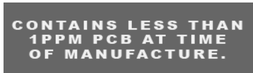
Figure 6.11. Nameplate, PCB statement
